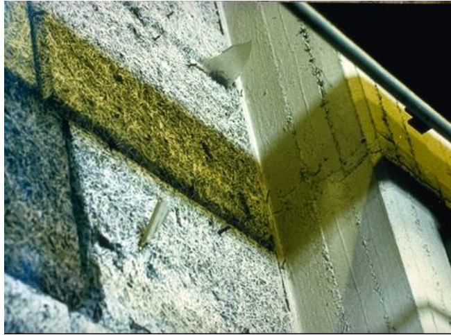
Figure 7. Glass fragments penetrated into a wall
