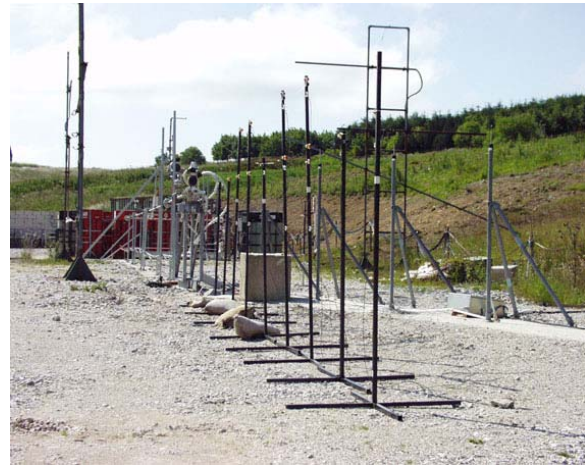
Figure 2(b). Oxygen depletion sensors for high pressure releases (towards release nozzle)
