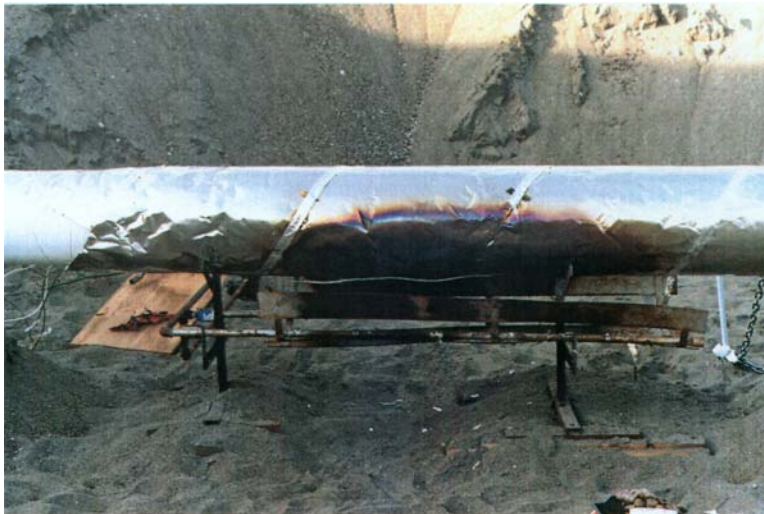
Figure 2: Photograph showing the intact condition of a composite tank wrapped with a ceramic blanket after having been exposed to an intense localized fire for 45 minutes.
