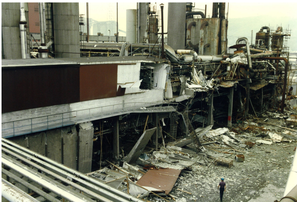
Figure 1. Photo of the factory building after the accidental explosion, taken by the investigation team photographer [5]. The photo shows the northern wall
