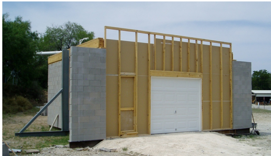
Hydrogen Release Garage Test Facility SWRI, San Antonio, TX
