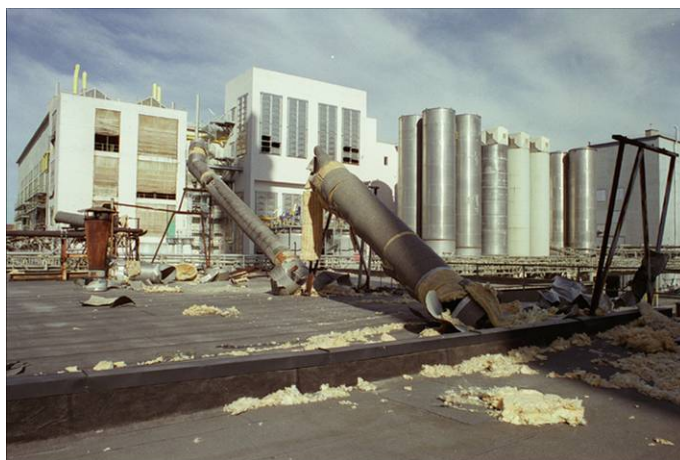
Figure 1: CO 2 line after hydrogen explosion
